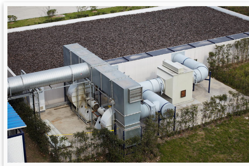
Waste air is bio-filtered through a bed of tree bark on the roof of a supplier facility. This is the final stage in the plant's comprehensive system for managing air emissions.
